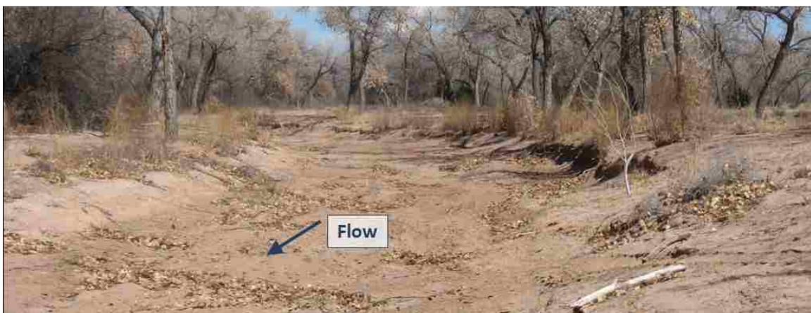
Figure 5-4: Bank Erosion along the Major Bend (02/2010)
